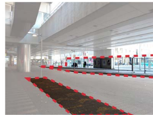
Faded wayfinding elements
