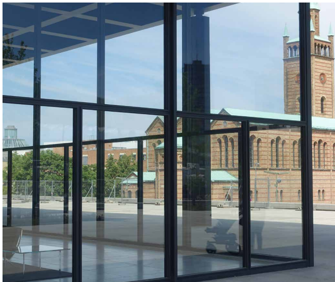
FIG. 5.39 New National Gallery, Berlin: original glazing (above) and three variants for the rehabilitation. In order to avoid glass breakage in the future, a double-thick laminated safety glass (2 x 12 mm) was used (second variant from above). The other two variants would have distorted the appearance of the construction too much. / Photo: F. May
