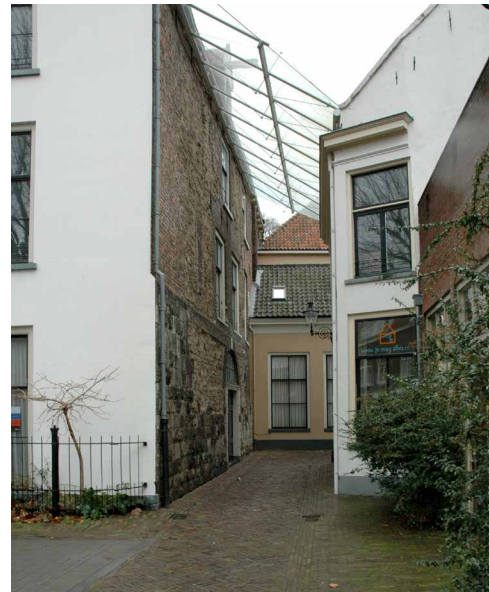
FIG. 4.11 A roof protection can be an alternative for a water-repellent treatment / Photo W.J. Quist
