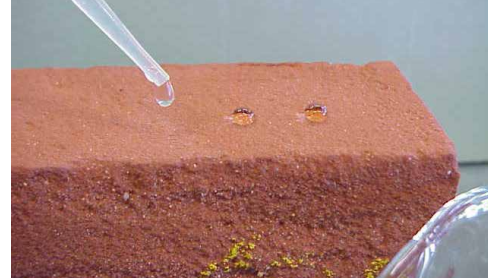
FIG. 4.19 Method for the assessment of effectiveness of water repellent treatment: beading effect / Photo: B. Lubelli
