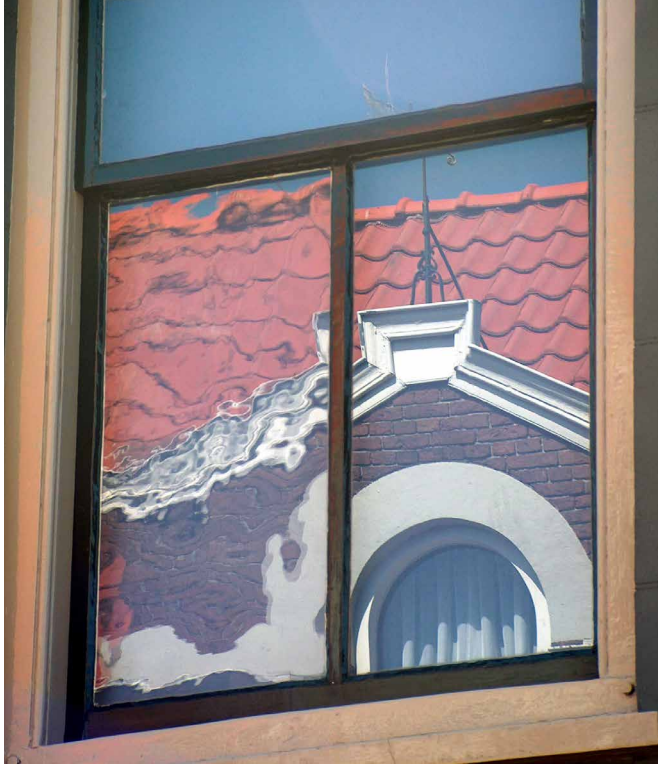
FIG. 5.26 Window with a historic irregular glass surface left and a new flat float glass surface right / Photo: H. v.d. Ven
