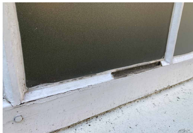
FIG. 5.18 Puttyed glass in wooden windowframe (in need of repair) / Photo: W. J. Quist
