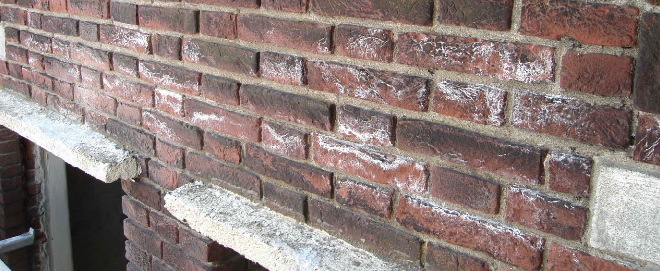
FIG. 4.28 Salt efflorescence, evidence of the presence of salts in the masonry, further confirmed by chemical analyses / Photo: B. Lubelli
