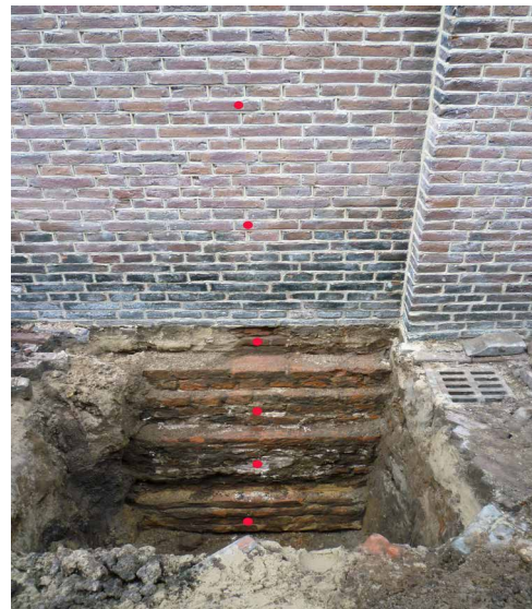
FIG. 3.13 Excavation of the ground around the foundation of the church and sampling, at different depths and heights in the wall along a vertical profile, for the measurement of the moisture content and distribution / Photo: B. Lubelli
