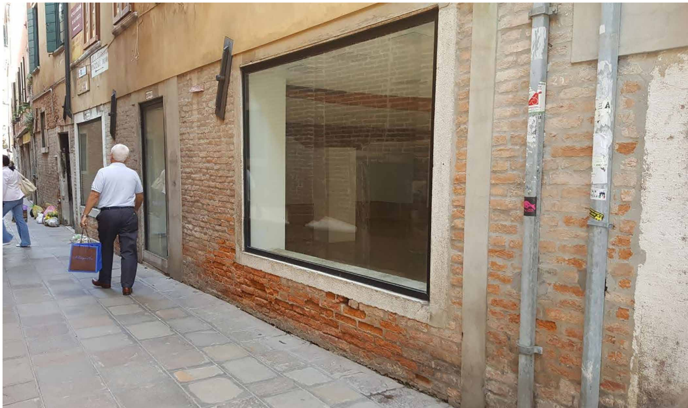
FIG. 3.1 Salt crystallization damage due to the presence of salts and rising damp, Venice, Italy / Photo: B. Lubelli
