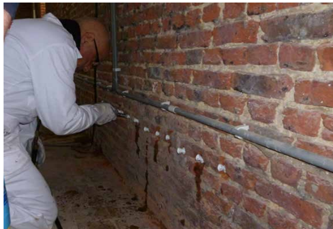
FIG. 3.5 Injection of a liquid product by means of pressure / Photo: B. Lubelli
