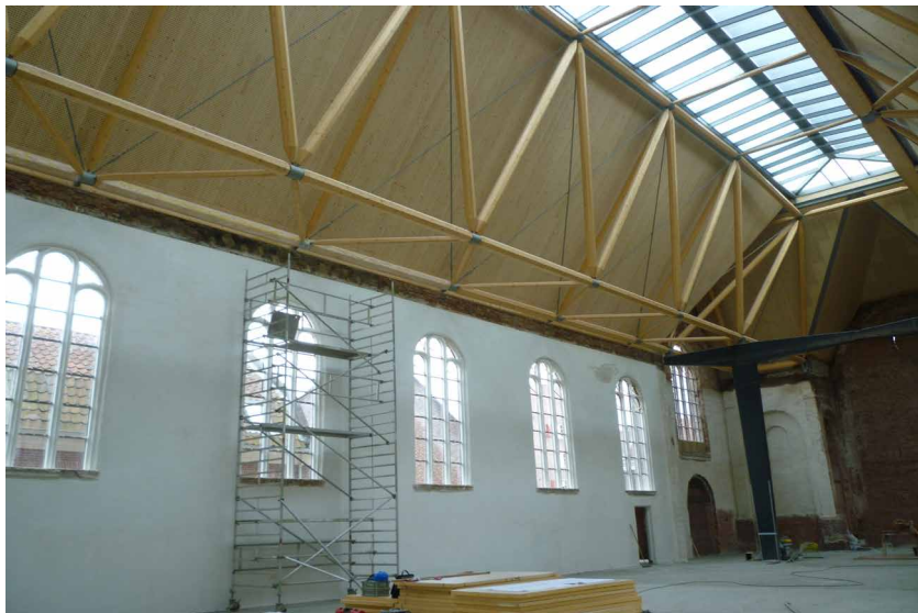
FIG. 3.12 Interior of the Elleboog church: water used to extinguish a fire had accumulated on the concrete floor and risen up in the wall, leading to a moisture content distribution similar to that observed in the presence of rising damp from groundwater / Photo: B. Lubelli
