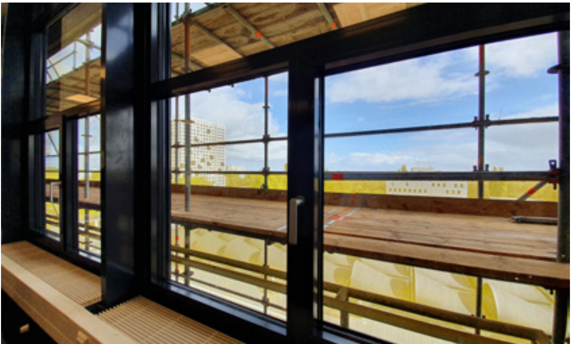
Façade Leasing “process” demonstrator project focusing on financial, legal, and managerial drivers and barriers to implementation. Built at the CiTG building, TU Delft, 2018-2019. Credits: Juan F. Azcarate-Aguerre, 2019
