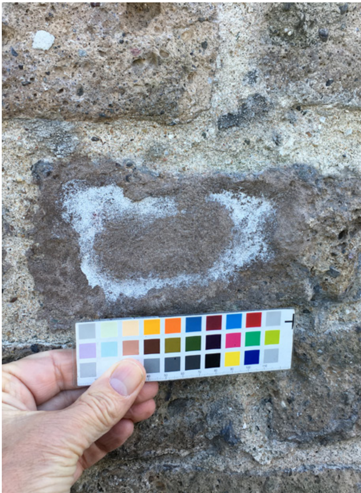
Salt efflorescences on repair mortar applied on tuff stone
