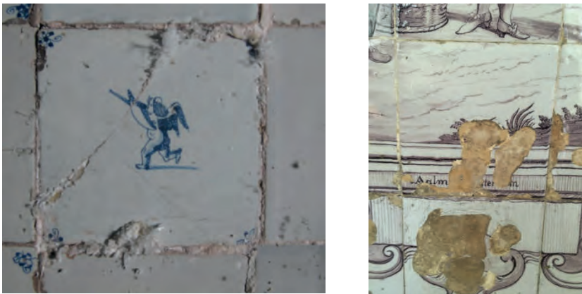
Figure 1: Salt efflorescence on the sides of a tile and along a breakage (left); blistering of the glaze (right).
