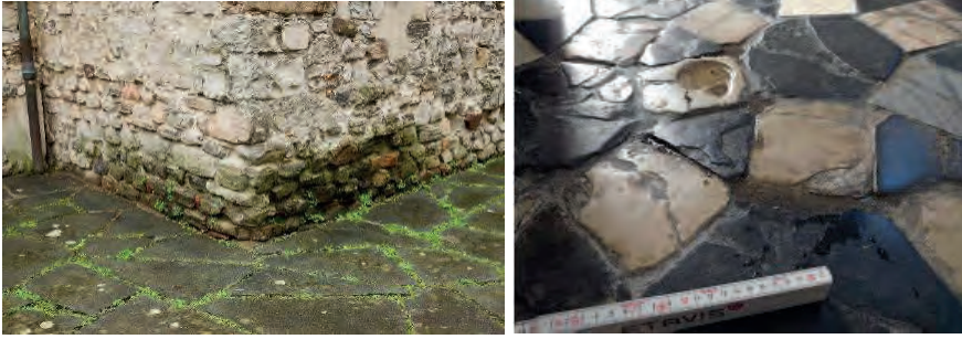
Figure 2: a) Phenomenon of capillary rising damp along the perimeter and biological colonization; b) Puddles of rainwater formed following water entry from the main door during heavy rains.
