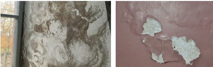
Figure 2: Typical salt related problems in a Neo-Gothic brick church where sodium sulphate is present. Left: Salt precipitation on the surface. Right: Flaking of paint.
