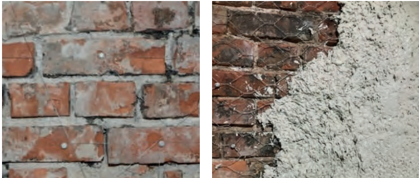
Figure 3: Stainless-steel wire (left) and chicken wire (right) acted as a reinforcing and plaster-bearing system. The hemp-lime had been applied here in a thickness of 10-30 mm directly against the brick wall.
