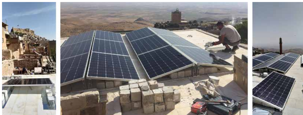
FIG. 9 Photovoltaic panels installed on the flat roof of Tamirevi. Source: KMKD Tamirevi Archives, taken by Süreyya Topaloğlu
