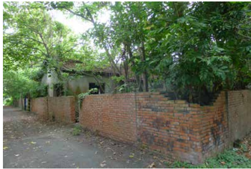
FIG. 15 Jianguo First Village in Yunlin County, one of 13 MD village cultural parks established by the Ministry of National Defense, awaits restoration. Source: Photographed by Szu-Ling Lin in 2016
