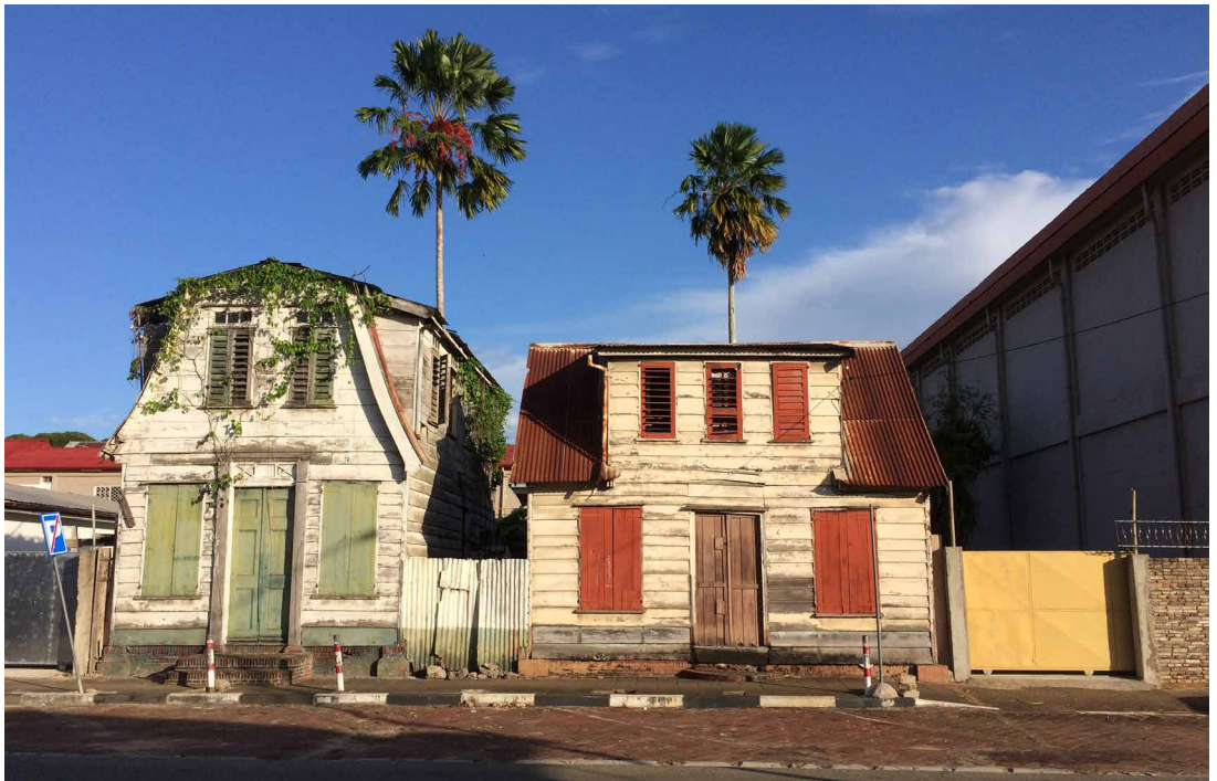
FIG. 2.3 Gebouwen in verval Examples of buildings in a state of decay
