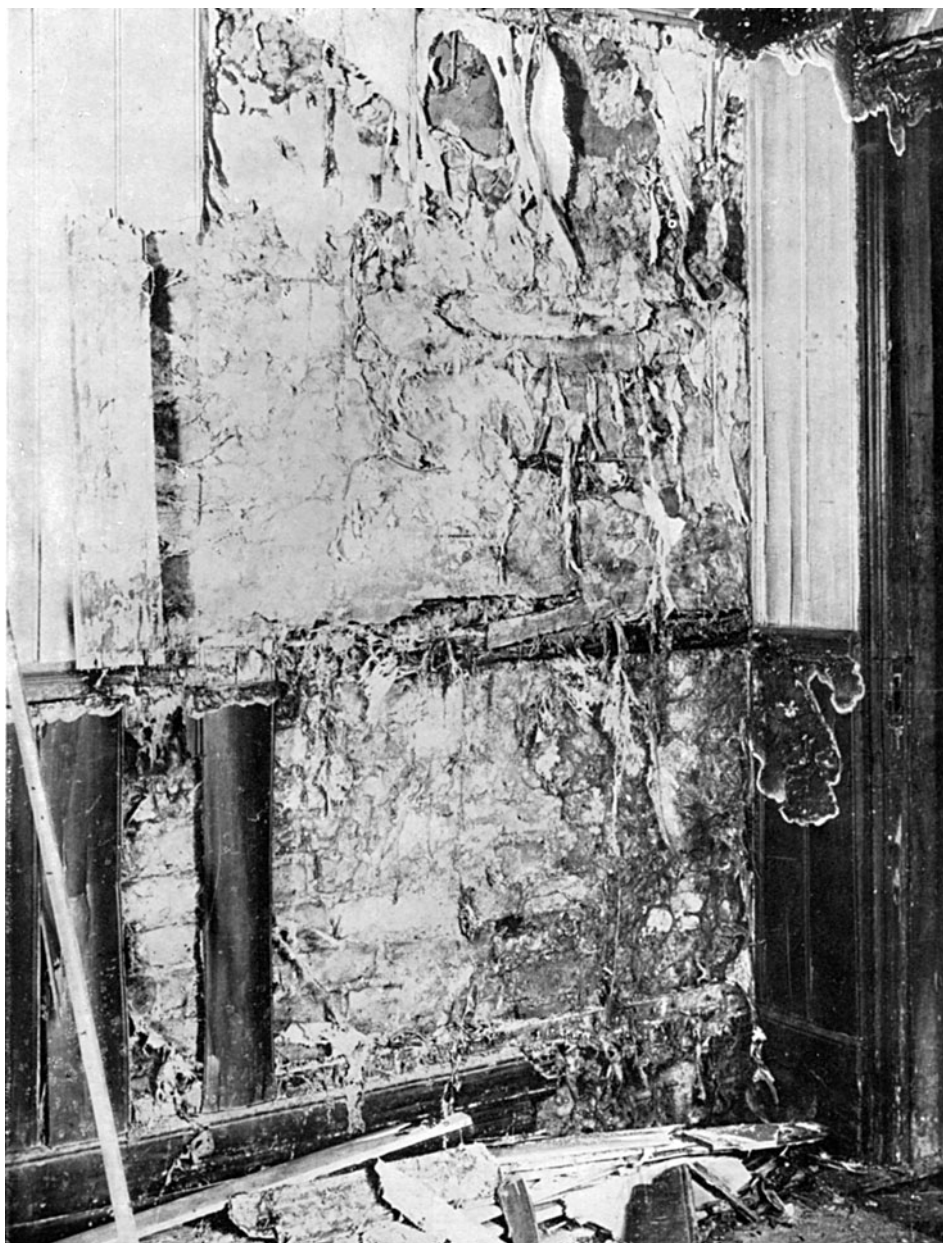
Dry rot caused by damp rising from the ground owing to the lack of a damp course
