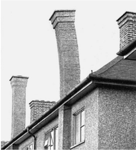
Chimney stack leaning owing to the chemical action of flue gases on the mortar
