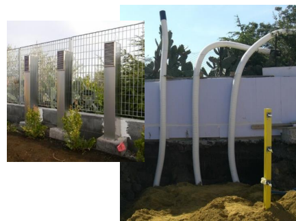
► Fig. 3: View of the earth to air heat exchanger (EAHE)
