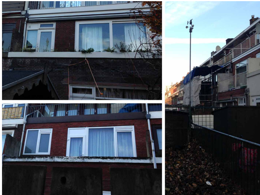
FIGURE 7.3 Maintenance problems in Oud Charlois, deterioration of balconies and façade. Source: author's pictures.
