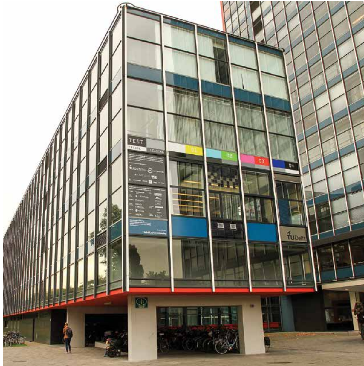
The Façade Leasing pilot project, installed on the EWI building at the TU Delft campus, Delft. Physical demonstrator of the state-of-the-art in façade-integrated technologies and decentralized services. Photograph: Marcel Bilow, 2016.
