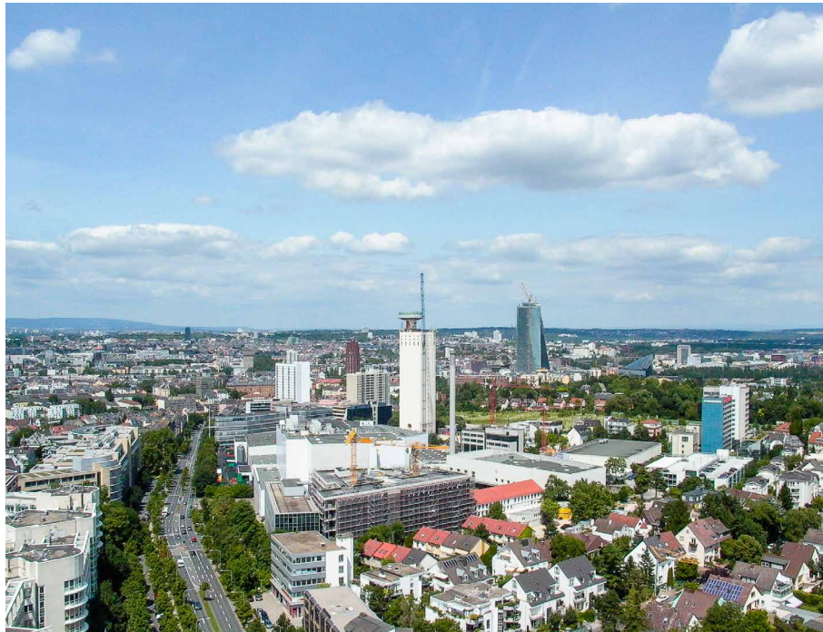
FIGURE 4.6 The Henninger Turm in Frankfurt Sachsenhausen four months after start of the dismantling process
