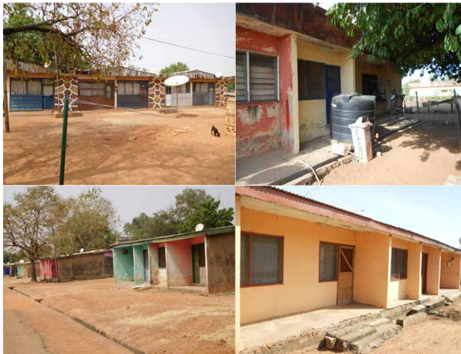
FIGURE 2.1 Conditions in public housing
