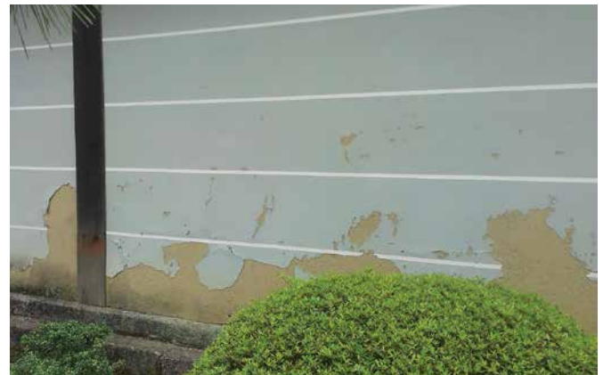
FIG. 14 Peeling of shikkui probably due to moisture infiltration from the bottom of the wall of a temple in Kyoto
