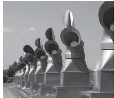
2 Application of venturi cowl rotating in wind direction; BedZED development in South London by the ZED factory (2002)
