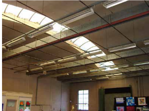
FIGURE 1.6 Roof lights illuminated the inner space of building Q in Woerden and partitioned the vault. Photo taken by author
