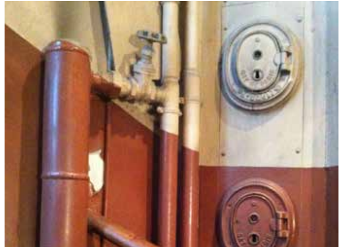
FIG. 3.42 Services in the servants' stairway of a multi-storied 19 th century apartment building, Paris / Marieke Kuipers
