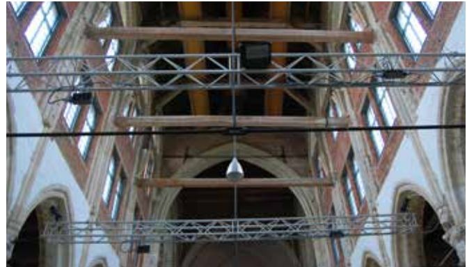
FIG. 3.3 The old structure of columns, vaults and beams, combined with new (reversible) elements of steel allow for the reuse of the Great Church of Veere as a flexible stage for cultural performances. Designed by Marx & Steketeer Architects / Marieke Kuipers
