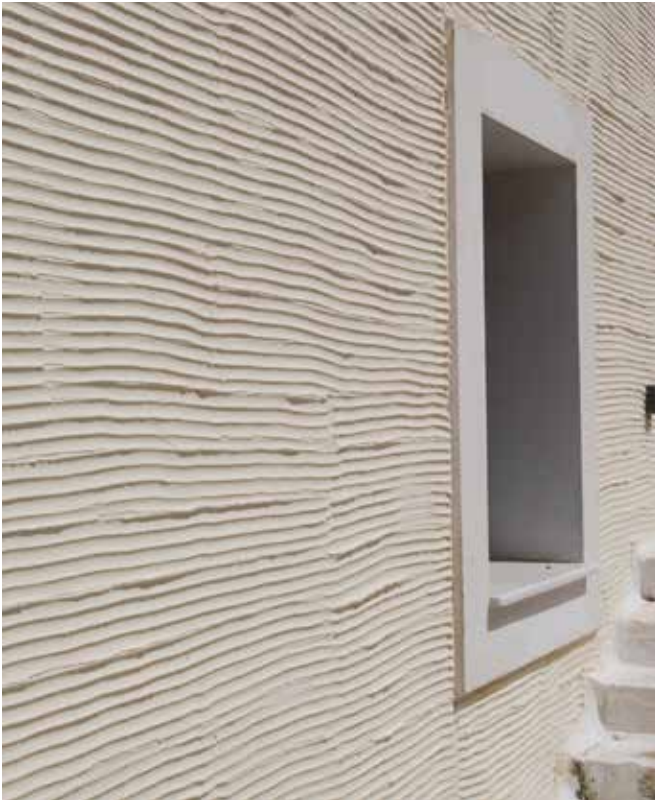
FIG. 3.13 Brushed plasterwork on a contemporary house on the Cycladic island of Andros, typical of the local tradition / Marieke Kuipers
