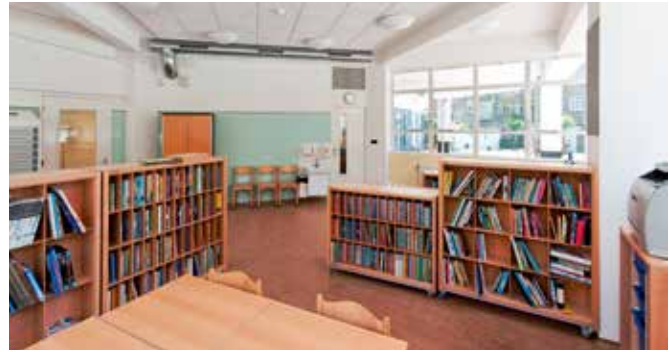
FIG. 5.31 Since classes are no longer taught outdoors, fresh air now is distributed through a small duct above the blackboard and then led through the overflow grate above the door to the staircase, which serves as a return duct / Tom Elst
