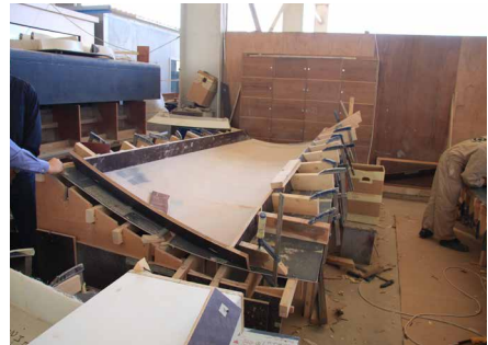
FIGURE 4.2 Wooden mould with a double curved surface. The double curvature is possible because of the big radii
