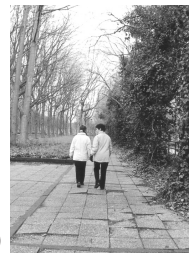
Fig.4-21 The effect of tree roots. Footpath near the Faculty of Architecture, Delft. (Photography by the author)
