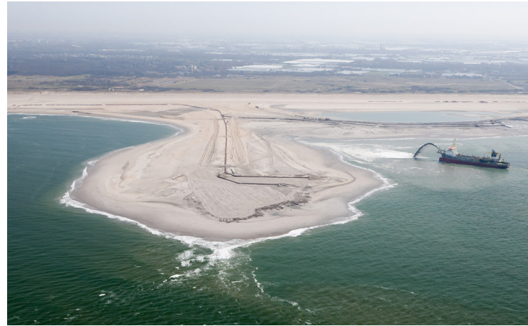
Figure 48. Construction of Sand Engine along the Dutch Coast 2011. (Photo Courtesy Rijkswaterstaat/Joop van Houdt)
