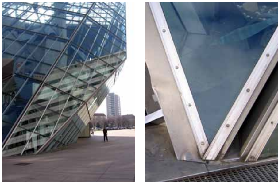
Figure 67 Non orthogonal façade construction, resulting in a joining detail that is inadequately solved with silicone.
