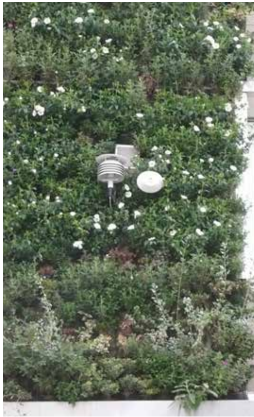
FIG. 2 Outdoor monitoring system after the installation of the vertical greening system
